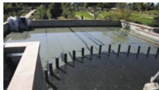
3 New roofing membrane is installed around wall posts. A water containment study is performed to ensure watertight seals.
