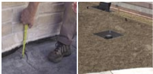
6 A gap is left under the wall so water can flow to roof drains.
