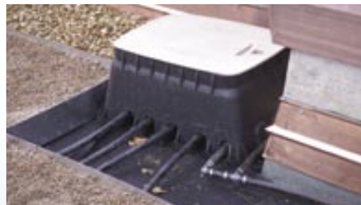
7 Irrigation system is installed for supplemental watering.
