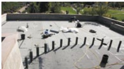
2 Prior to installing the new roofing membrane, wall posts are attached to the roofing structure to properly contain the Bison deck system.
