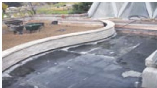
10 Rooftop space is ready for pedestrian decking with Bison Wood Tiles and Deck Supports system.
